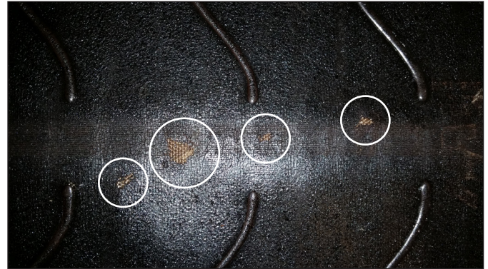
Failed Belt Wrap - Worn.
